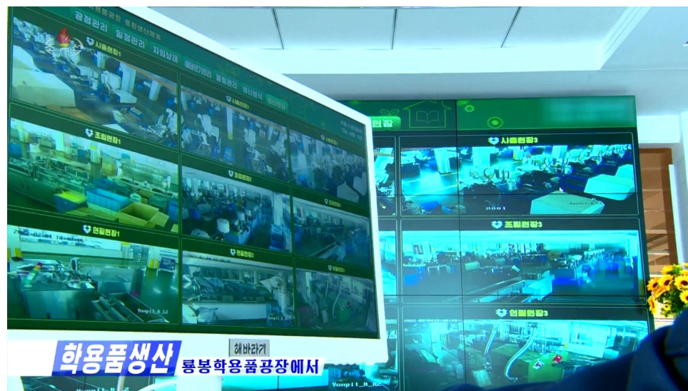
Figure 20. The control room at the Ryongbong School Supplies Factory, seen on Korean Central Television on February 7, 2022.
