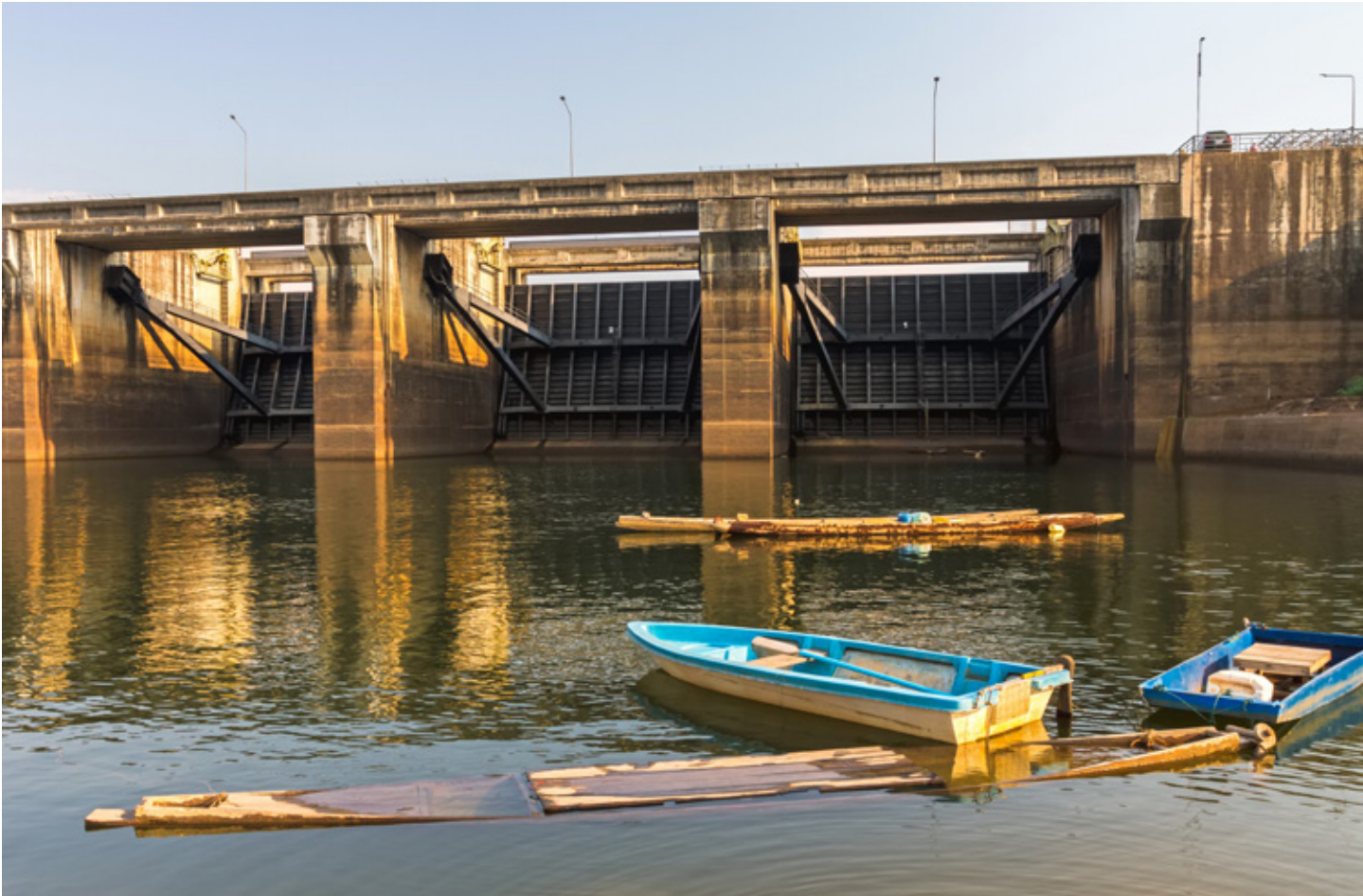
The Pak Mun Dam, constructed on the Mun River, tributary of the Mekong River, in Ubon Ratchathani Province, Thailand.
