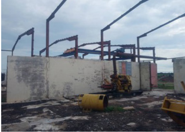
Bentiu power station, destroyed in the civil war. Thudan Gai Majiok
