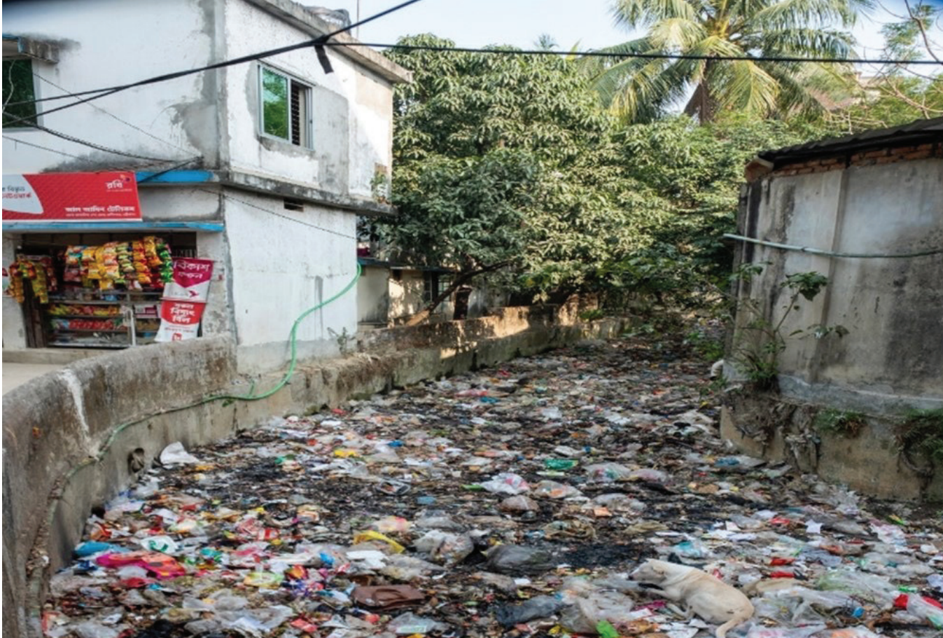
Drainage channel in Chattogram clogged with solid waste, 2022
