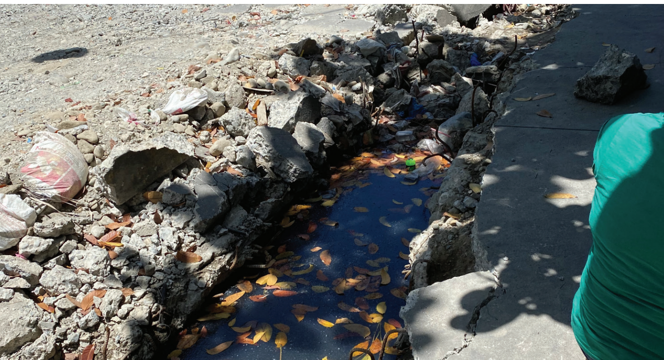
City canals clogged by plastics and debris. Photo: Sabrina Escalona.
