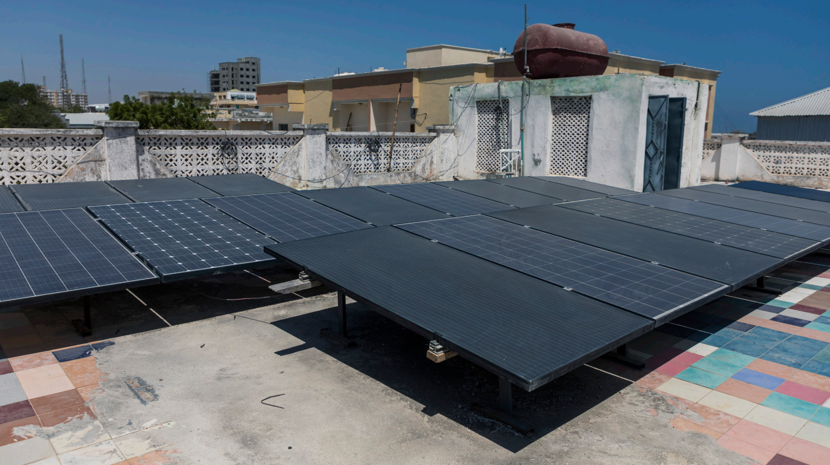
Tamarso Energy Plant, Mogadishu, Somalia Photo: Osman Nor
